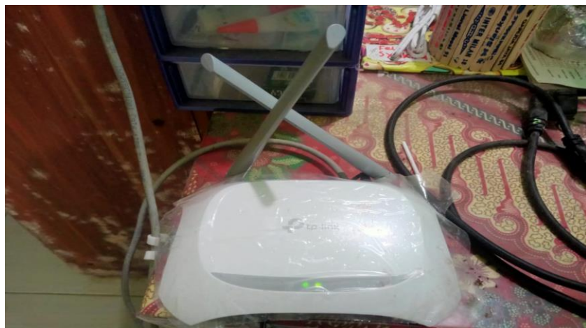
Gambar 4.14 instalasi jaringan internet (Wifi)
